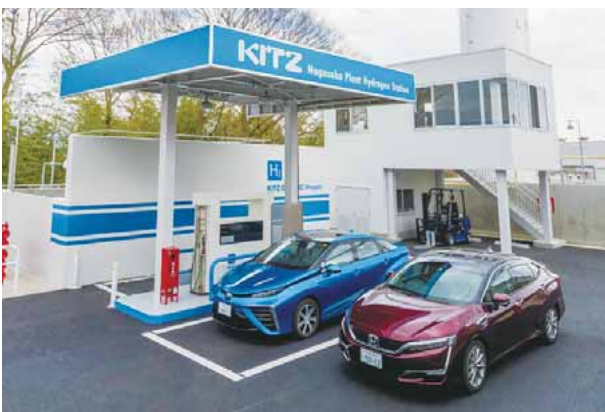
KITZ Nagasaka Plant's hydrogen station (internal use)
